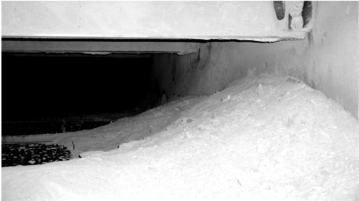
Figure 5: Typical Ash Accumulation in SCR Catalyst Boiler Side
